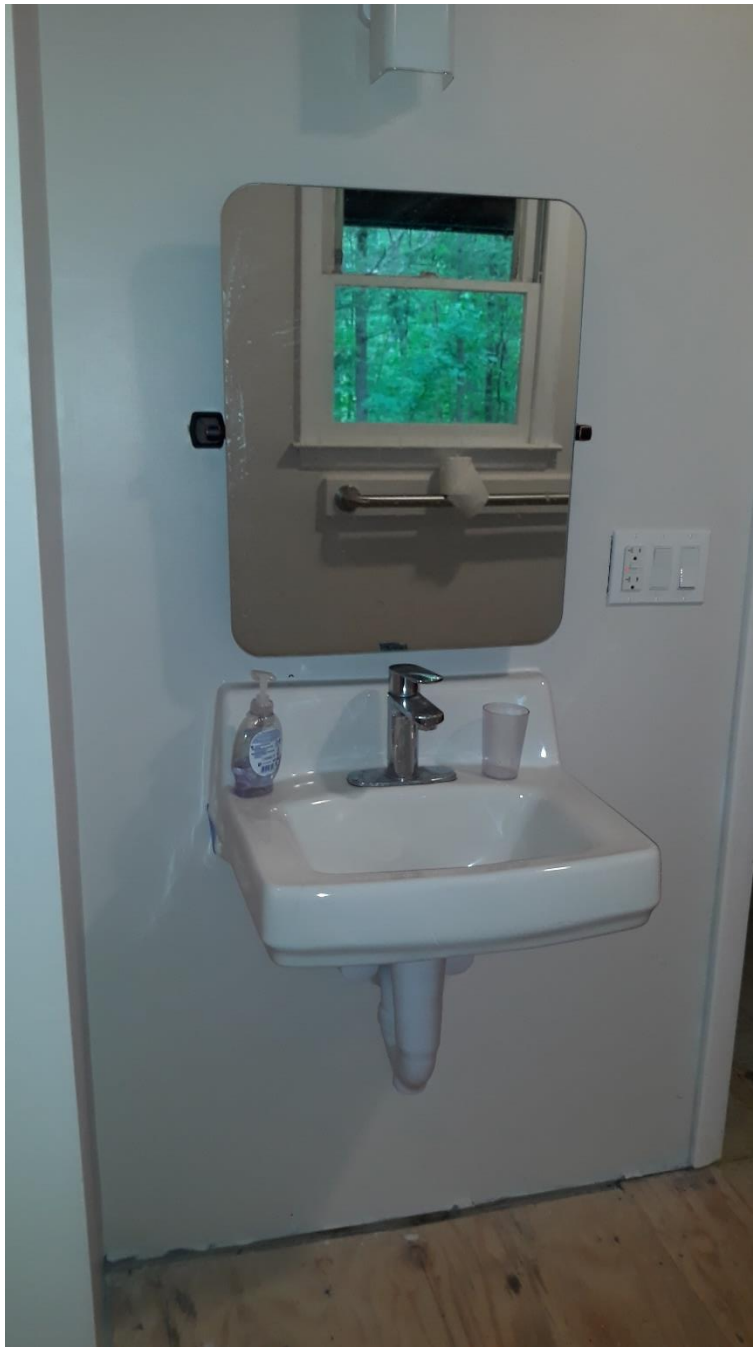
NEW ADA COMPLIANT SINK & MIRROR
