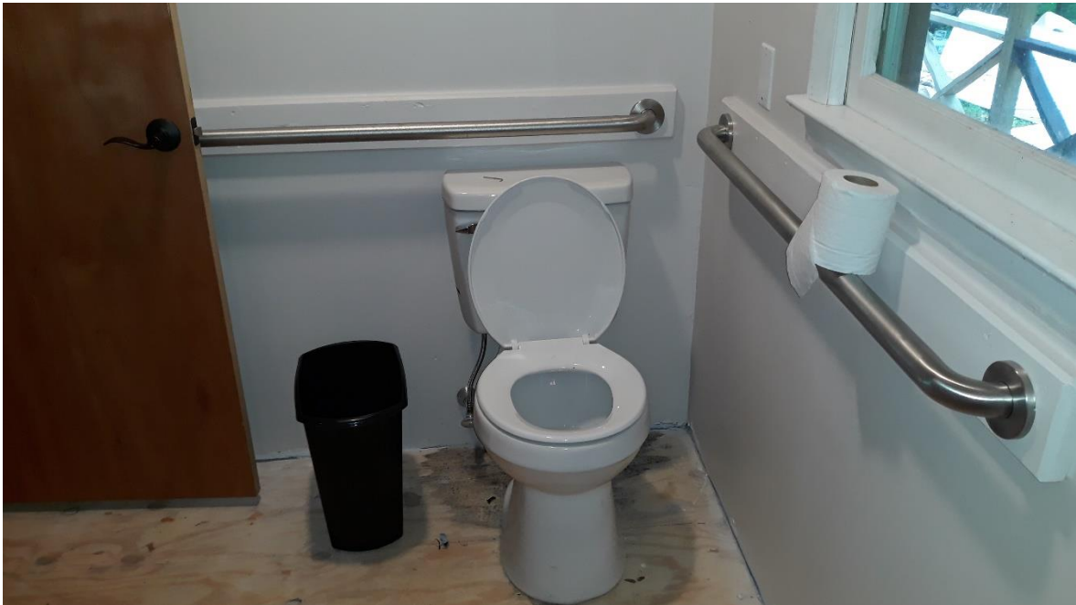
NEW ADA COMPLIANT LAVATORY
